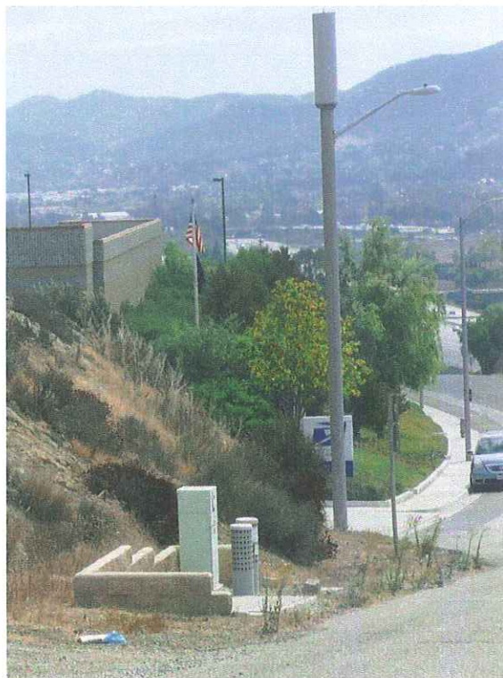
6 - Facility enclosed in cylinder on top of light pole in Newbury Park. Note regular light pole to right of one in foreground. The accessory equipment is underground, except for electrical meter and vents.
