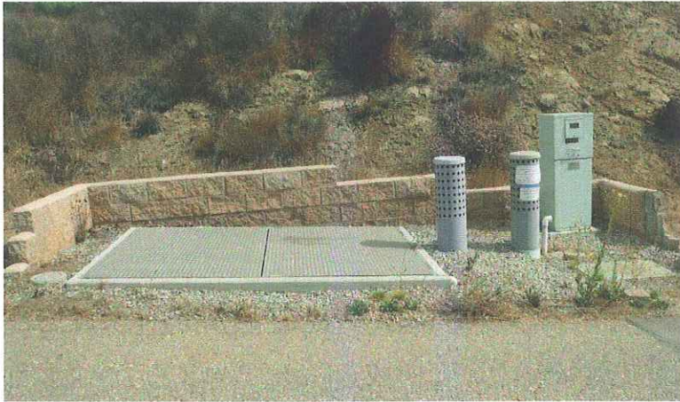
7 – Detail of accessory equipment underground, except for electrical meter and vents. Retaining wall protects structure.
