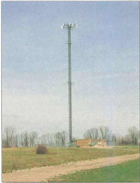
9 – Example of guyed tower – not in City.
