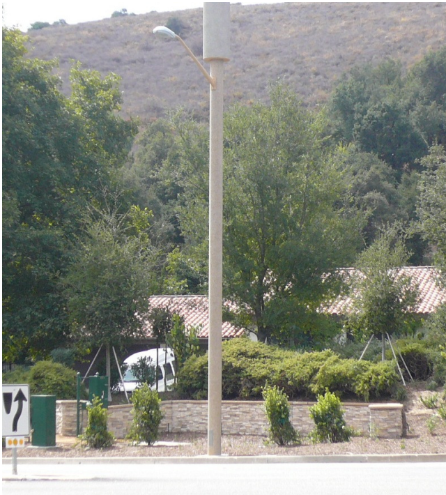
8 - Facility enclosed in cylinder on top of light pole in ROW in City of Thousand Oaks. The accessory equipment is underground, except for electrical meter and vents, and includes decorative wall and landscaping.
