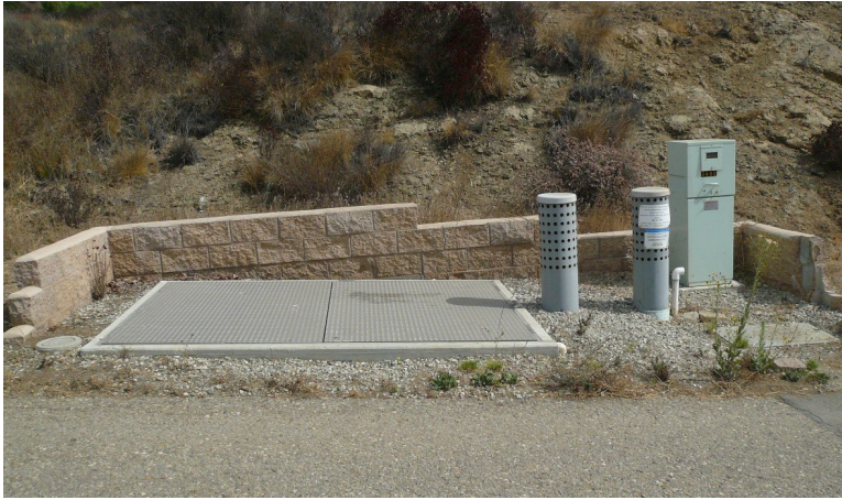
7 – Detail of accessory equipment underground, except for electrical meter and vents. Retaining wall protects structure.
