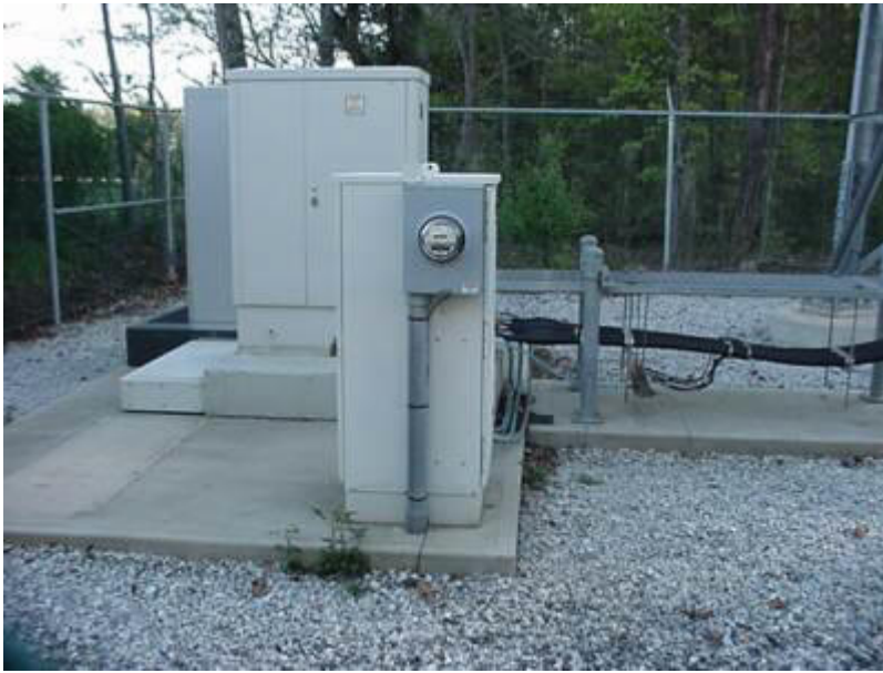
9 – Accessory equipment above ground – not in City.
