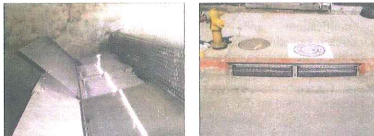
Figure 60: Catch Basin Grates and Filters
