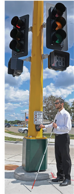
An accessible pedestrian signal
