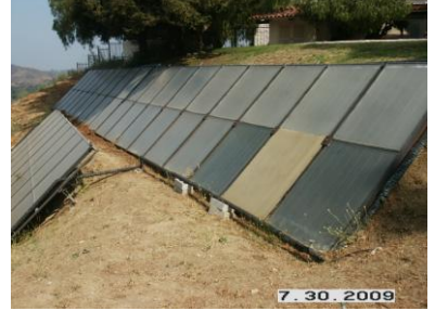
Ground-mounted solar panels
