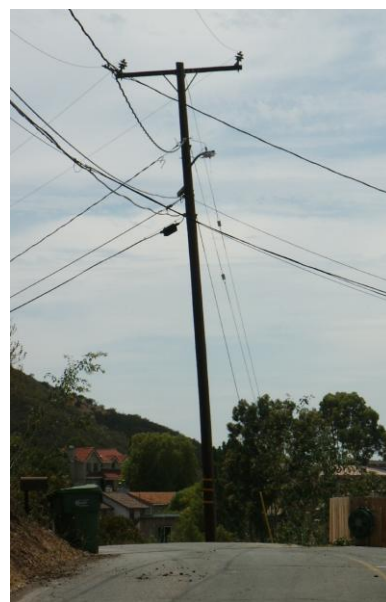
Power lines along Laura La Plante Drive
