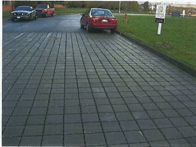
Figure 3. Pervious pavers used in the roadway of a neighborhood development in Wilsonville, OR (Source: Abby Hall, US EPA).
