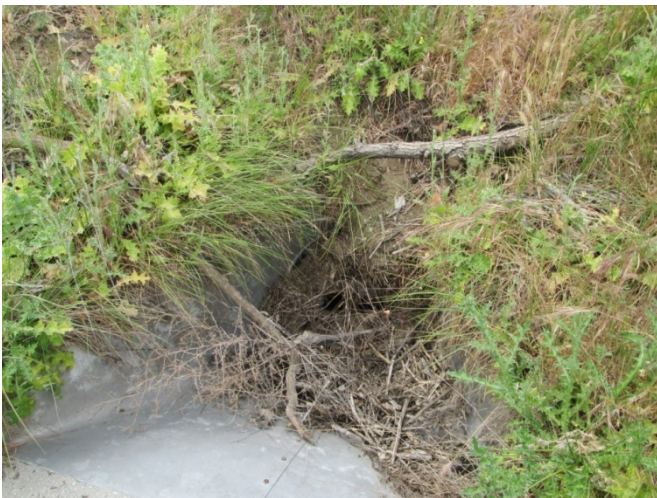
View of a large storm drain at the center of the Property
