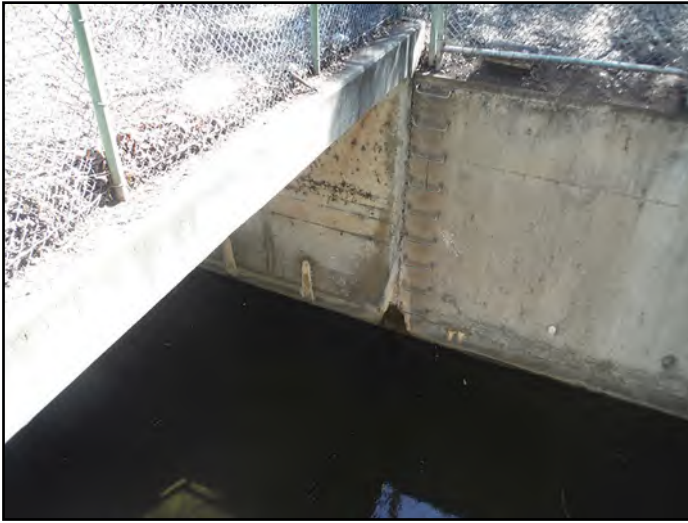
Photo 2A – Lindero Creek flows in a closed and an open concrete box culvert beneath the site. The open section of Lindero Creek in the southwestern portion of the site is shown.
