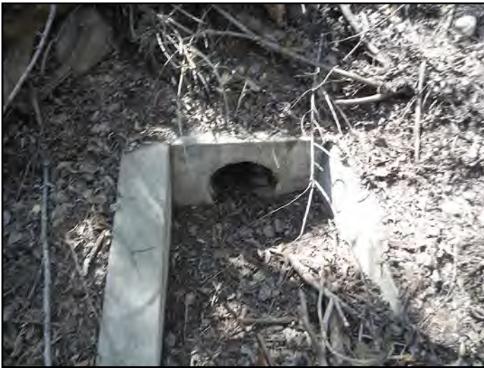
Photo 2C – This small on-site culvert inlet discharges to the jurisdictional stream wetland located near the northeastern site boundary.
