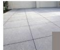
11 CONCRETE PAVING FINISH: MEDIUM BROOM, SAW CUT COLOR: NATURAL GRAY BY: NEW CONSTRUCTION
