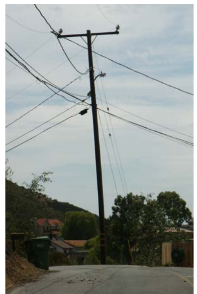
Power lines along Laura La Plante Drive
