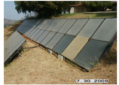
Ground-mounted solar panels
