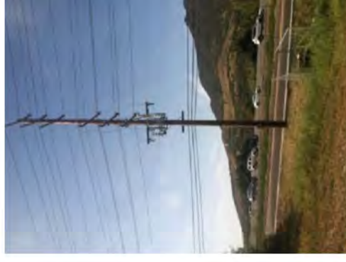
Photograph 6. View of the pole mounted transformer adjacent to the southeastern corner of the subject property, facing south.
