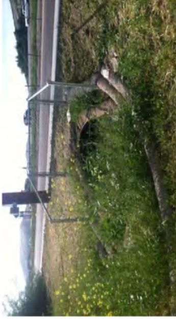
Photograph 5. Drainage culvert on the southeastern corner of the subject property, facing south.
