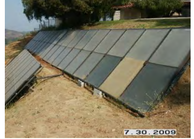
Ground-mounted solar panels
