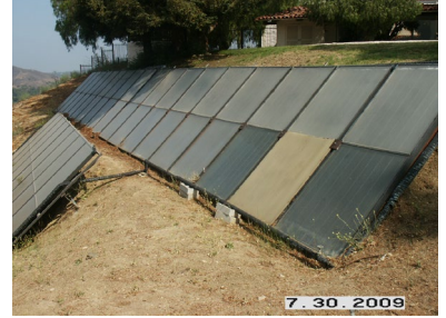
Ground-mounted solar panels
