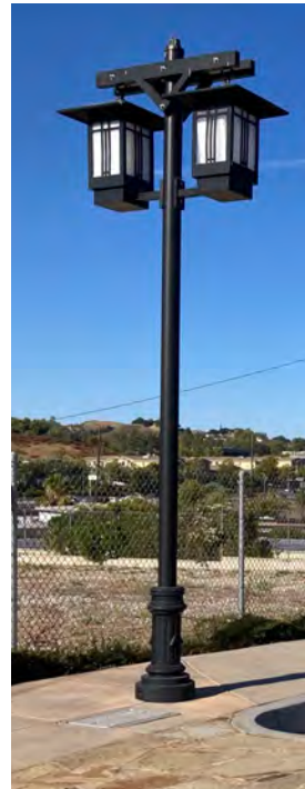
Street and Pedestrian lights
