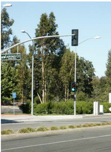
Optimizing traffic signal timing can help improve traffic flow and reduce delays
