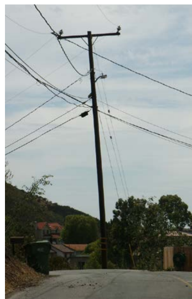
Power lines along Laura La Plante Drive
