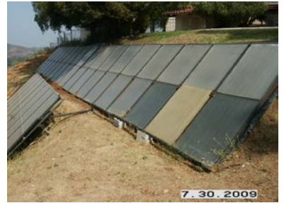
Ground-mounted solar panels
