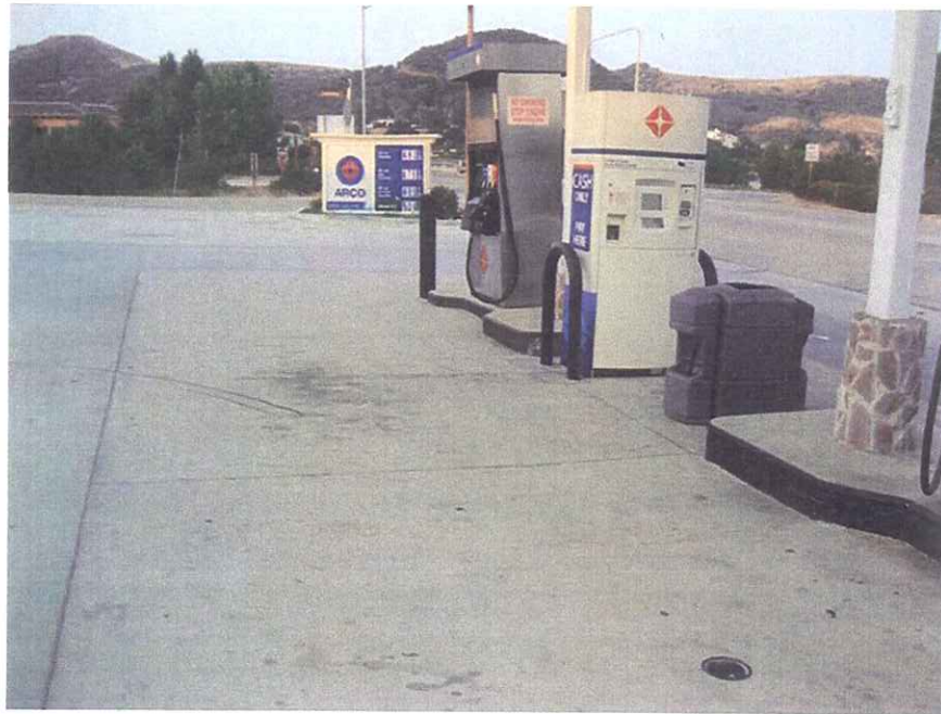
#3 Looking south along Palo Comado Canyon Road – note the proximity of the pumps to Palo Comado Canyon Road..
