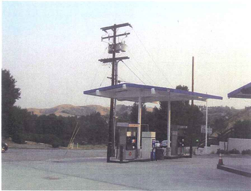
#5 Note the pole-top transformers along Palo Comado Canyon Road.
