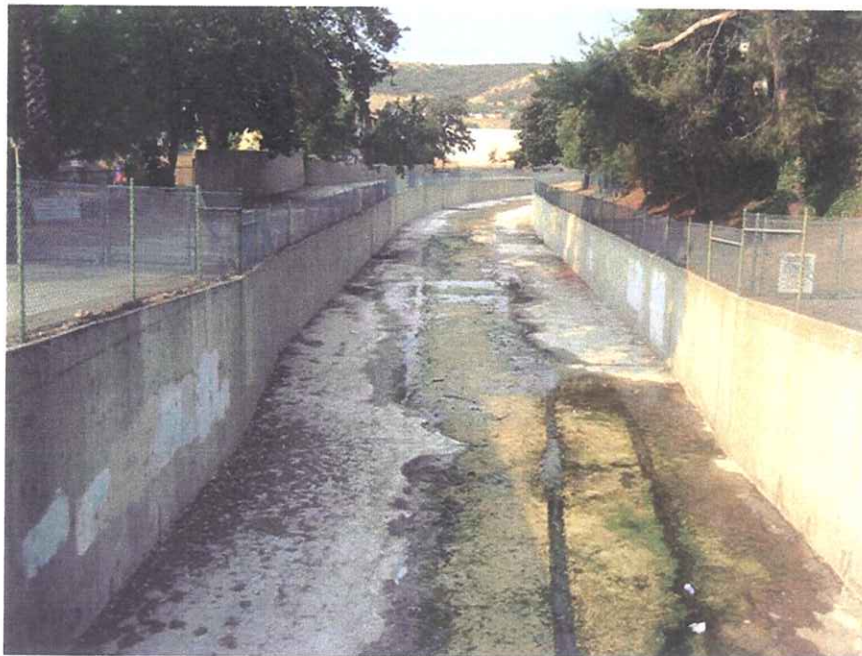
#18 The concrete lined wash north of U.S. 101 and west of Chesebro Road.
