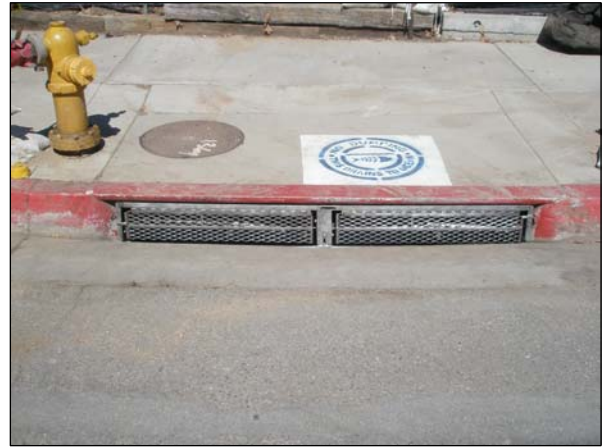
Catch Basin Filters located at Driver Avenue
