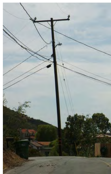
Power lines along Laura La Plante Drive
